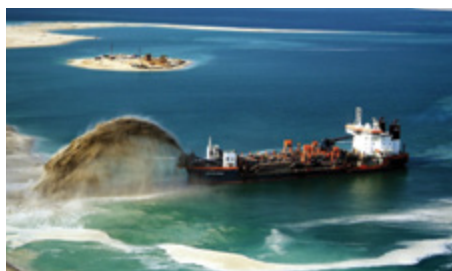
The Trimble Marine Construction systems provide the 3D position of the dredge head and displays it with the channel design. Precise information gives marine operators "eyes under water", to see exactly where material should be dredged.
